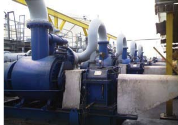
Houttuin two-screw pumps
