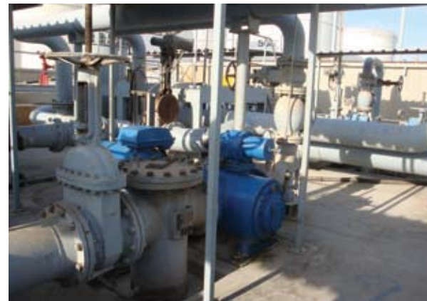
Houttuin two-screw pumps
