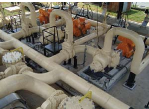
Houttuin two-screw pumps
